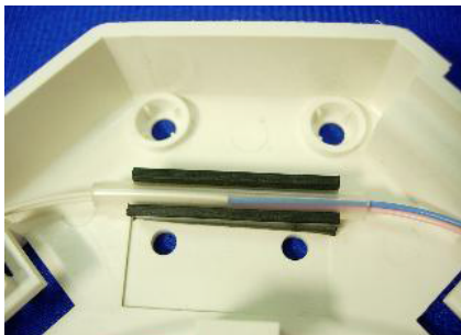
Step 4: Splice suitable pigtails to the cable fibers, cover the spliced section with the protection sleeve and place it in the rubber retainer as shown.
